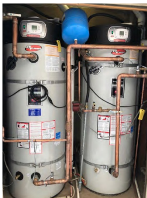
(2) Condensing Water Heaters
