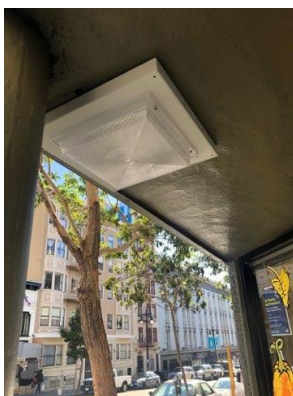
New LED Fixture (Front Entryway)
